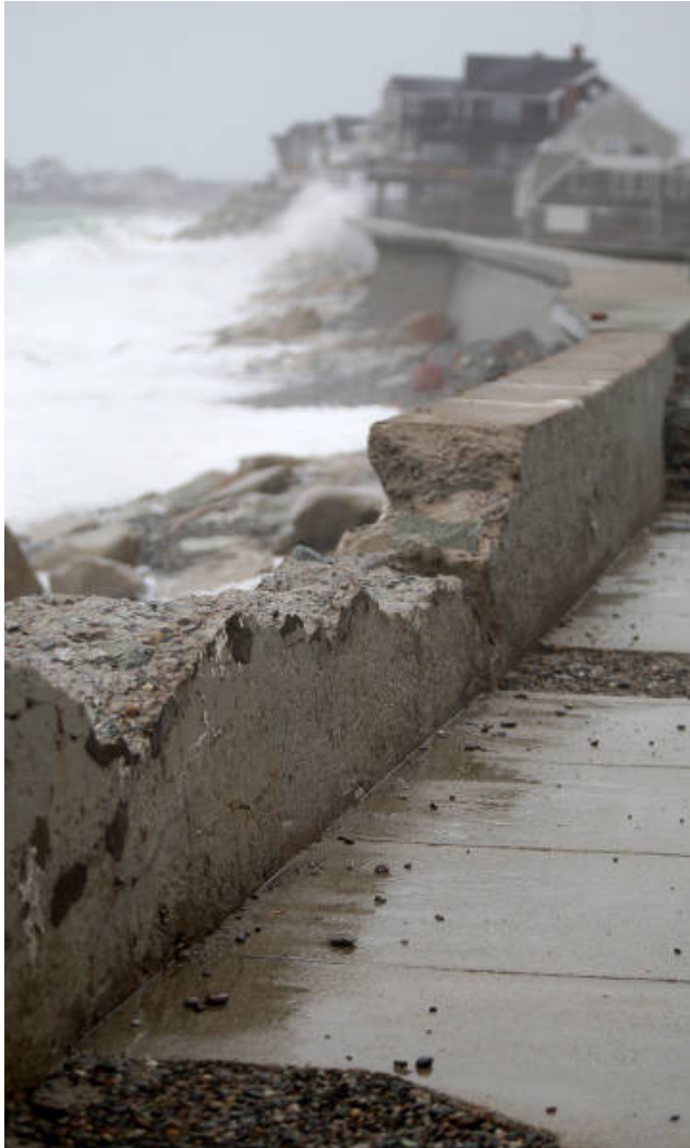
Plate 1. . Seawalls deteriorate with age and damage from storm events.
